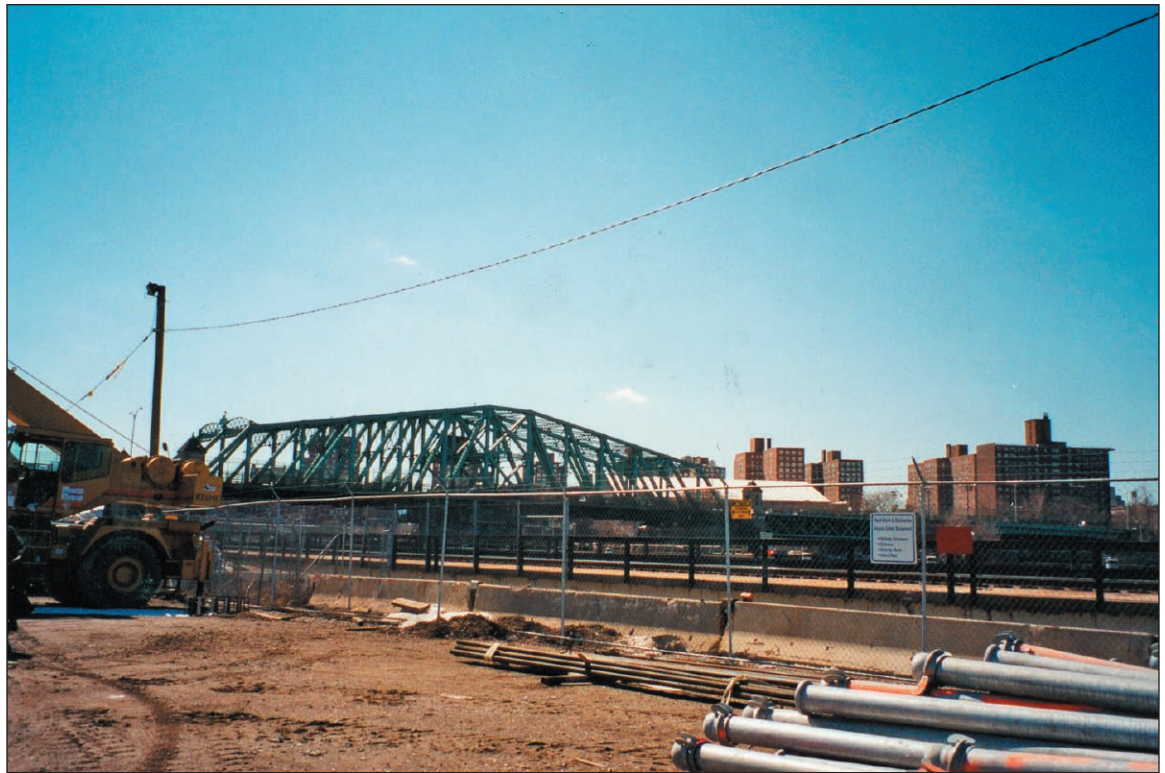
View south from area south and west of the Bronx Terminal Market including the 145th Street bridge and the Manhattan (Harlem) skyline
