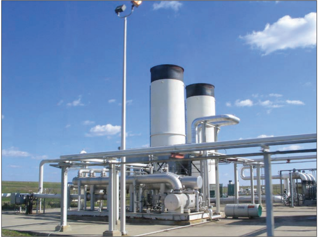
Flare Station, North Mound 9
