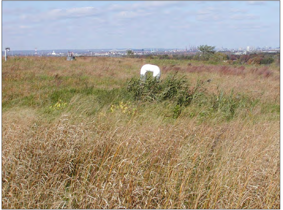
Typical methane ventilation pipe 11
