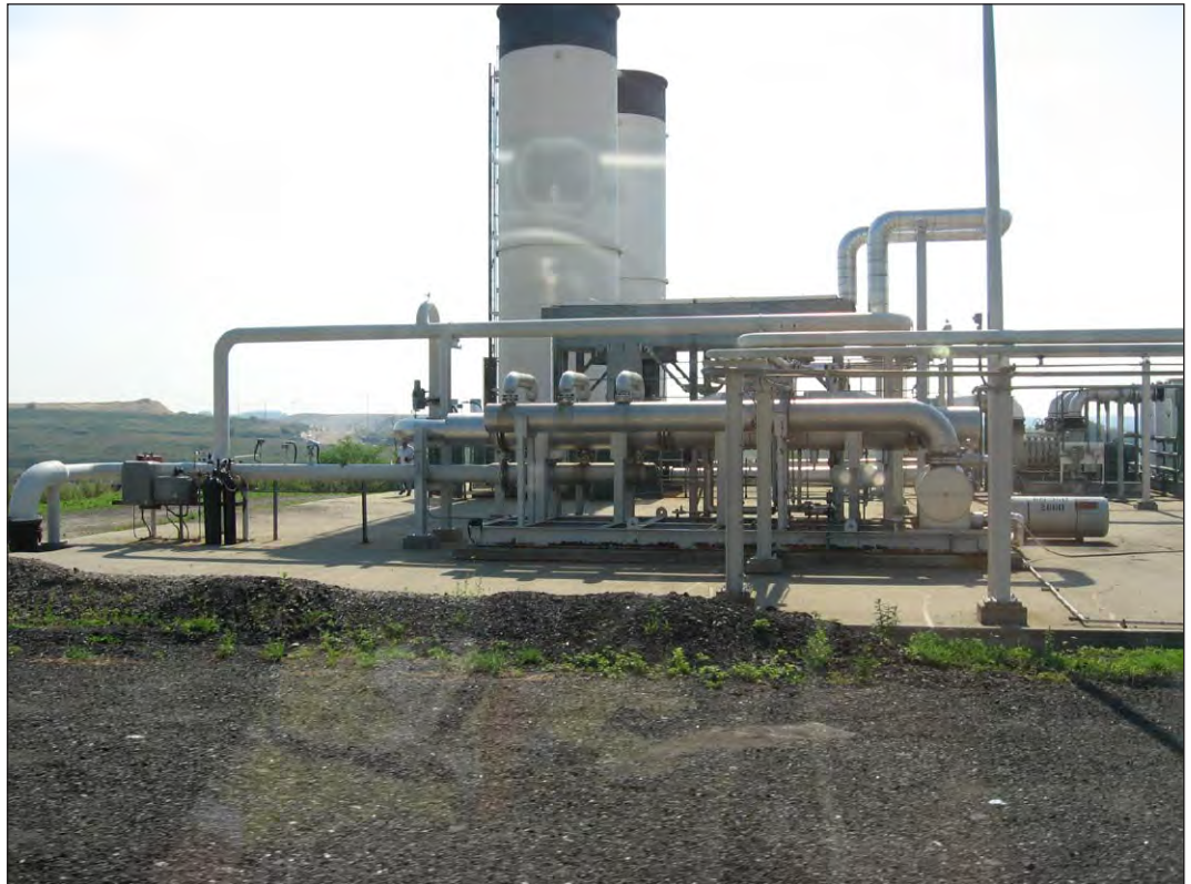
Flare Station on North Mound, looking southeast 2
