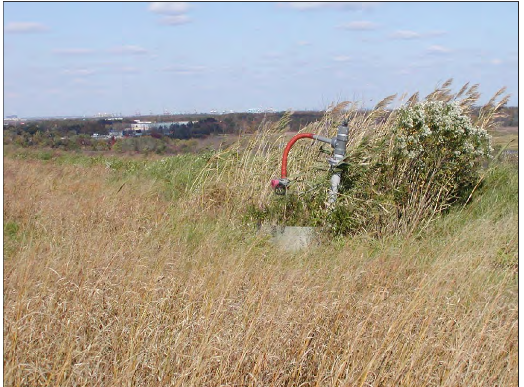
Typical utilities on North Mound 12
