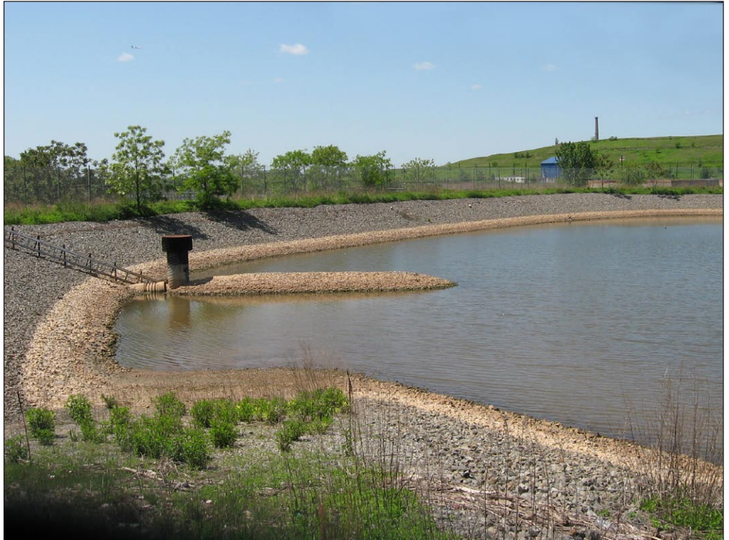
Smaller of the two stormwater basins located at the Convergence of Main and Richmond Creeks 9
