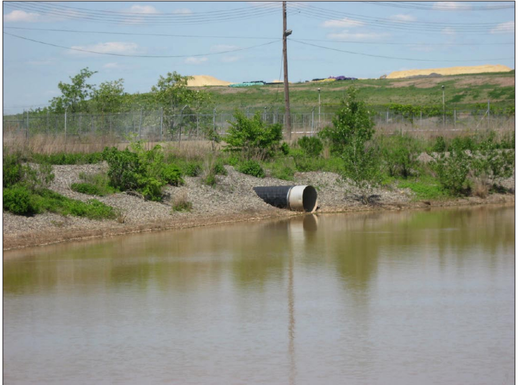
Large stormwater management basin at the Convergence of Main Creek and Richmond Creek 7
