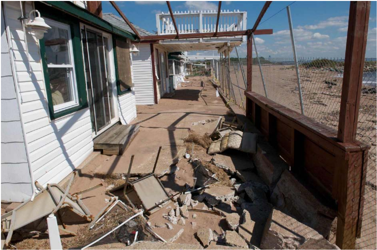
Photo 5: View looking north on Cedar Grove Beach, with damaged bungalow facing the ocean.
