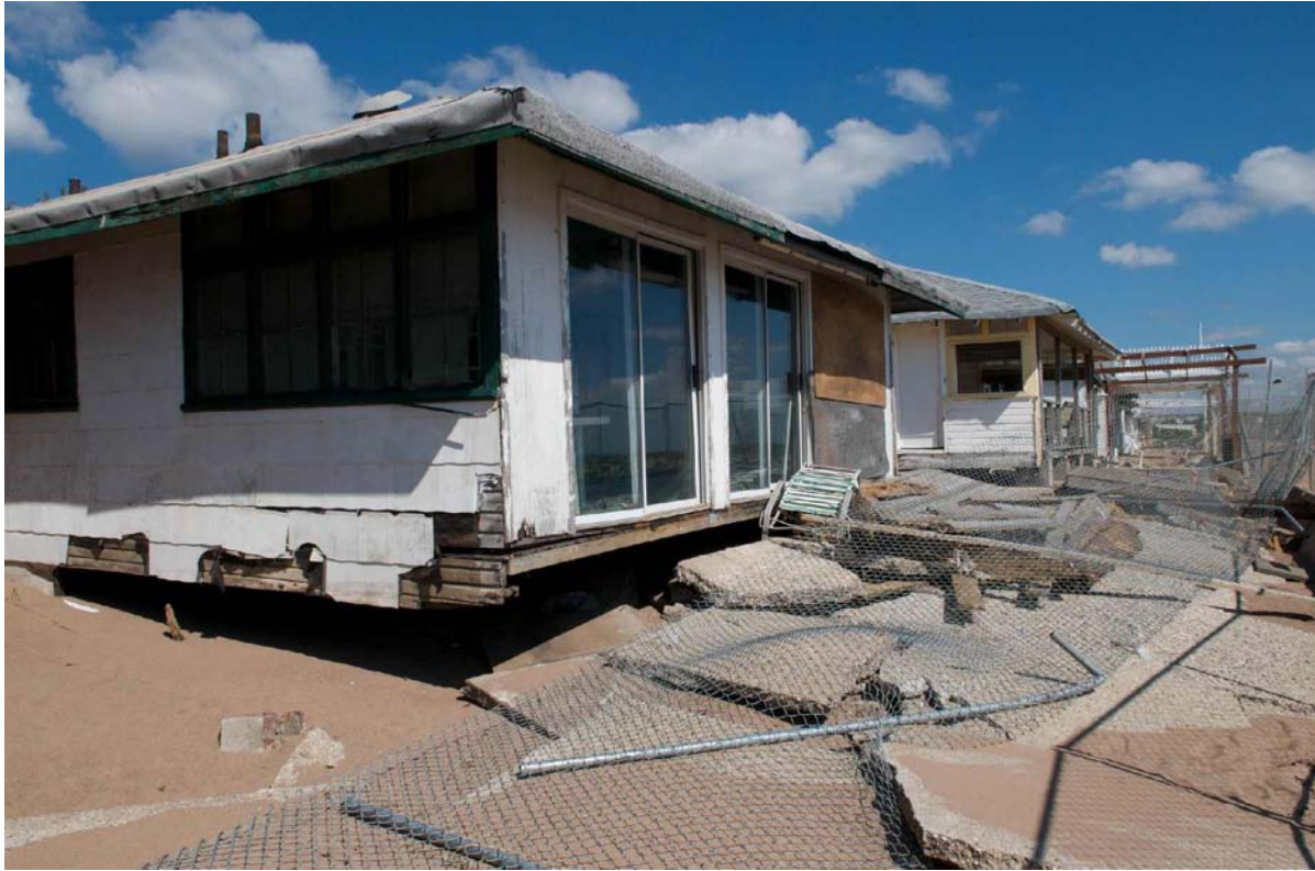
Photo 1: View looking north on Cedar Grove Beach, with damaged bungalow in foreground.
