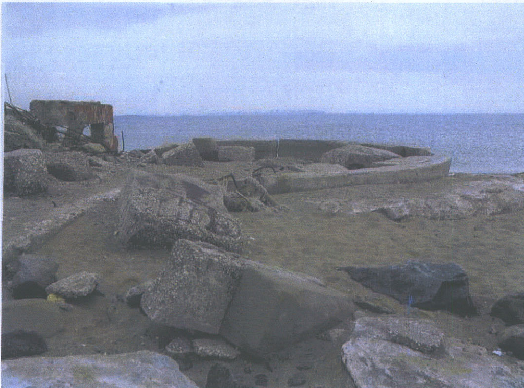
Photograph 12: Foundation remains and debris on the beach off Ebbitts Street and Cedar Grove Court. View looking northeast.
