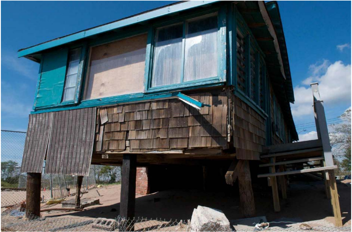
Photo 3: View looking southwest on Cedar Grove Beach, with damaged bungalow in foreground.
