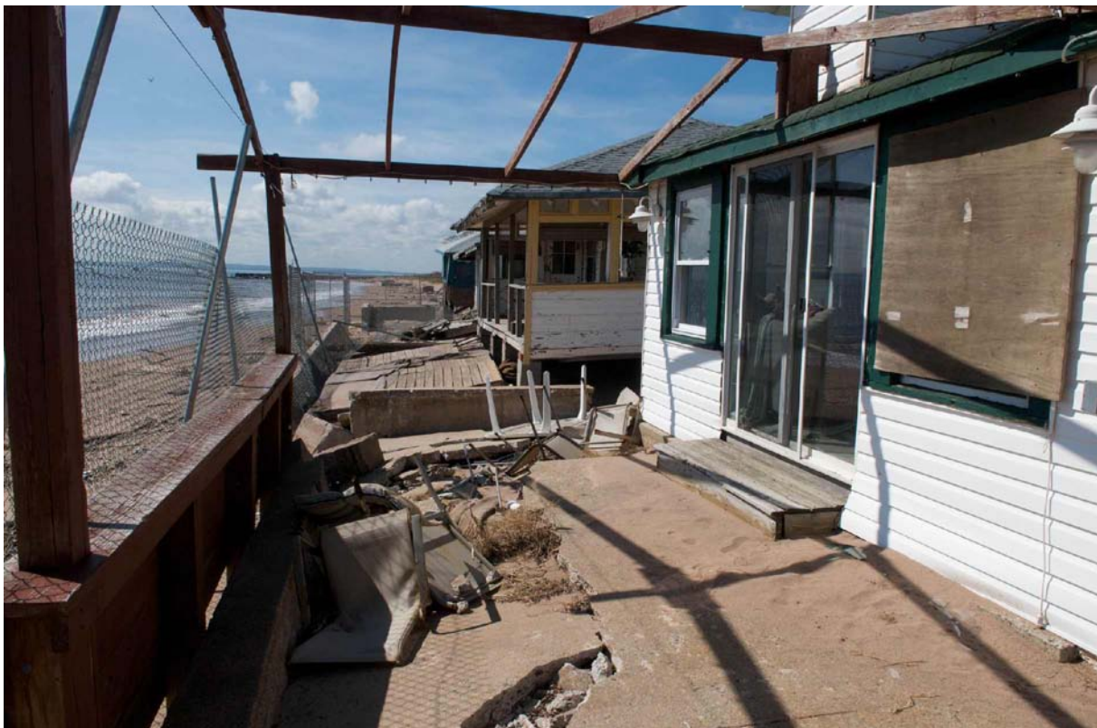
Photo 6: View of damaged bungalows looking south along Cedar Grove Beach.
