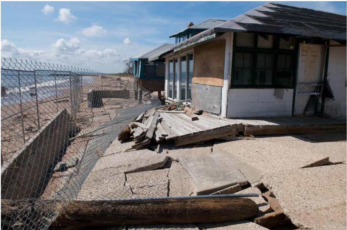
Photo 4: View of damaged bungalows looking south along Cedar Grove Beach.
