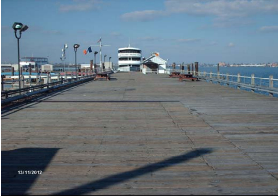
Fig. 7. Image of Pier 1 post-Hurricane Sandy provided by the Subrecipient.
