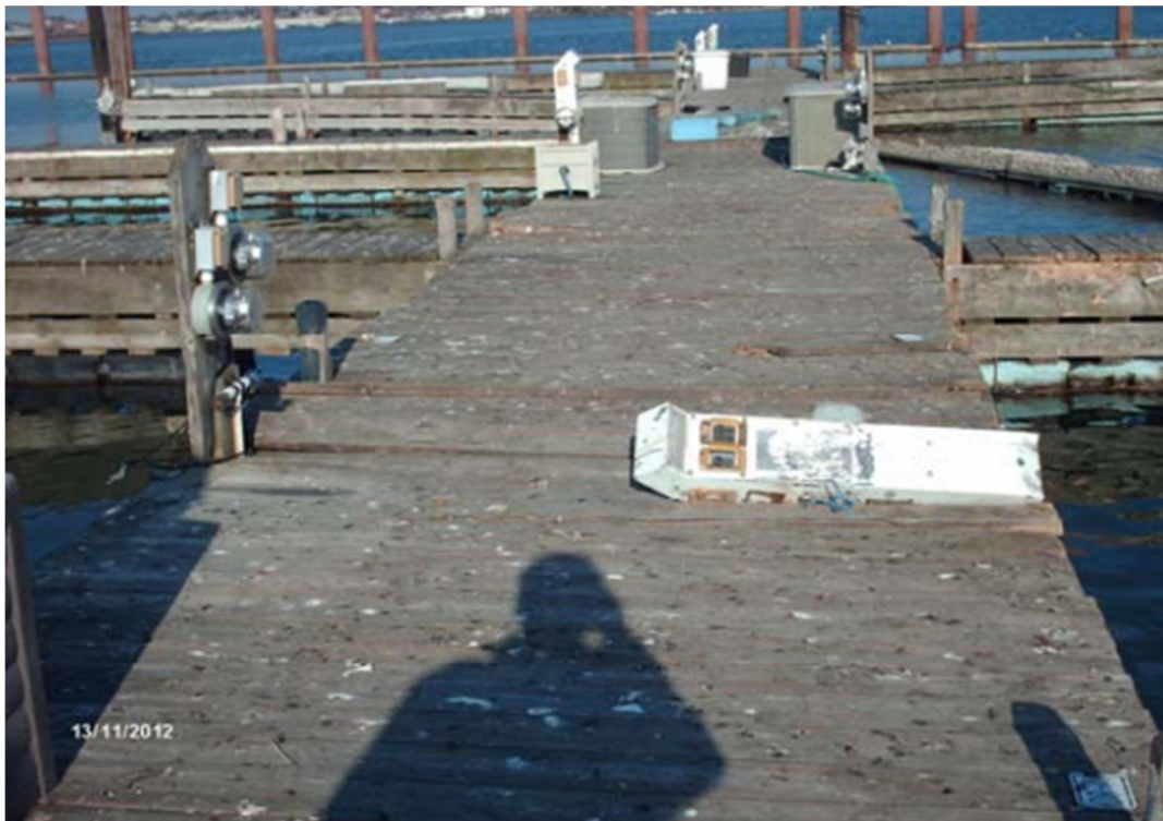
Fig. 10. Image of Pier 1 post-Hurricane Sandy provided by the Subrecipient.
