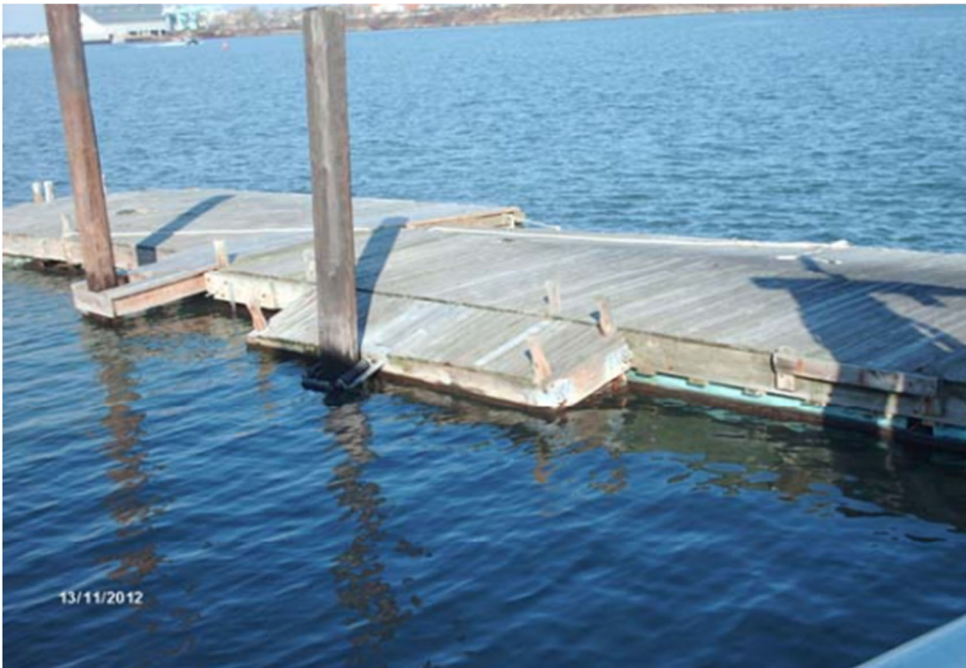
Fig. 8. Image of Pier 1 post-Hurricane Sandy provided by the Subrecipient.
