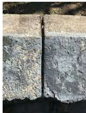
15 UPWARD-FACING JOINT IN GRANITE COPING STONE
