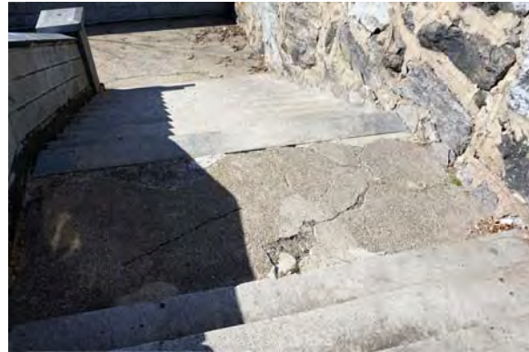
4 FAILED PREVIOUS REPAIR ON LANDING
