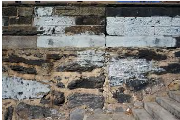
10 GRANITE STONE WALL CRACK
