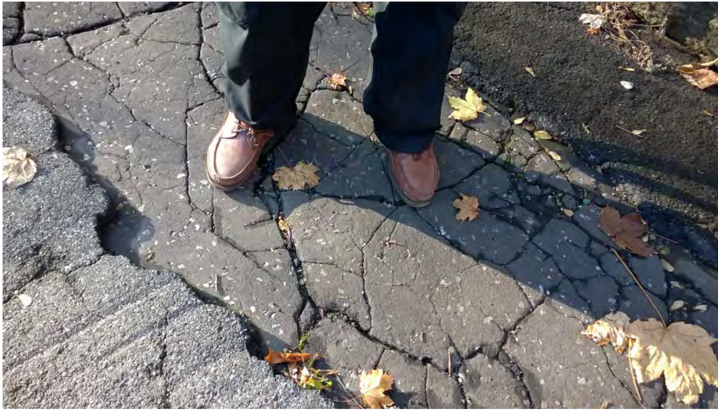
11 - Poor pavement condition is typical along this northern section.
