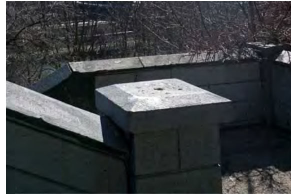
7 MISSING LIGHT FIXTURE
