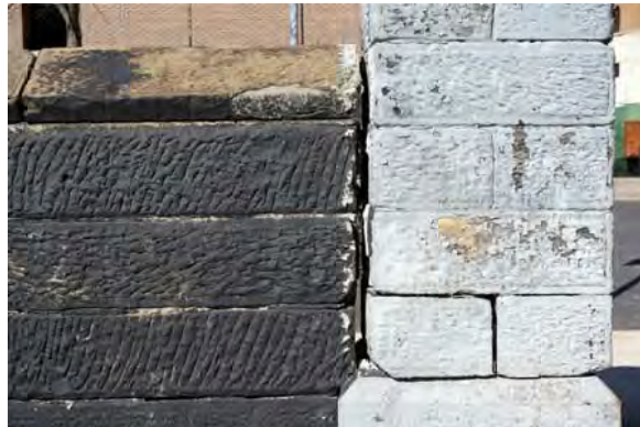
2 GRANITE PIER & PARAPET DISPLACEMENT
