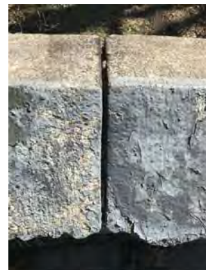
15 UPWARD-FACING JOINT IN GRANITE COPING STONE
