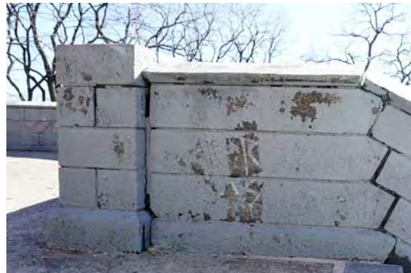
6 MISSING GRANITE COPING
