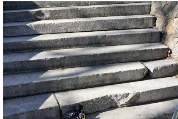
5 CHIPPED / DAMAGED GRANITE STEPS
