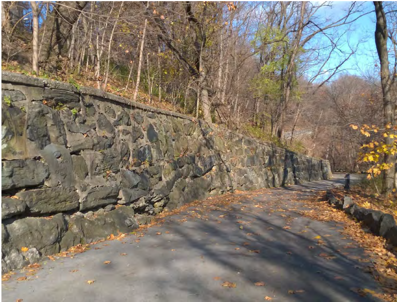
7 - Stone retaining walls are a blend of dry-laid and mortared components and may include integrated rock outcrops.
