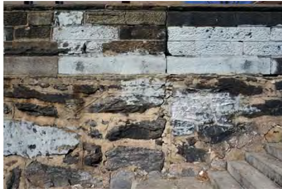
10 GRANITE STONE WALL CRACK
