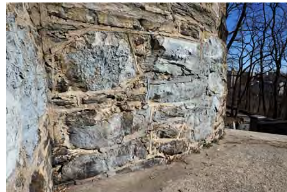
14 GRAFFITI AND PAINT
