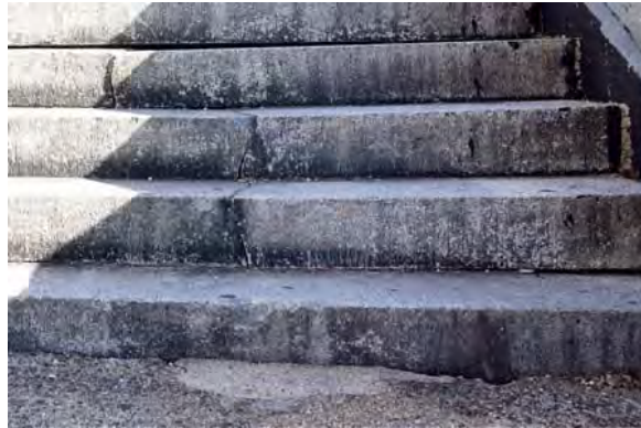
1 CRACK ON GRANITE STEP
