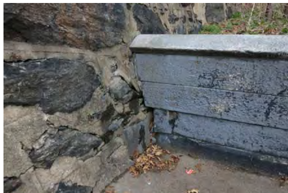
12 VOIDS & MATERIAL LOSS
