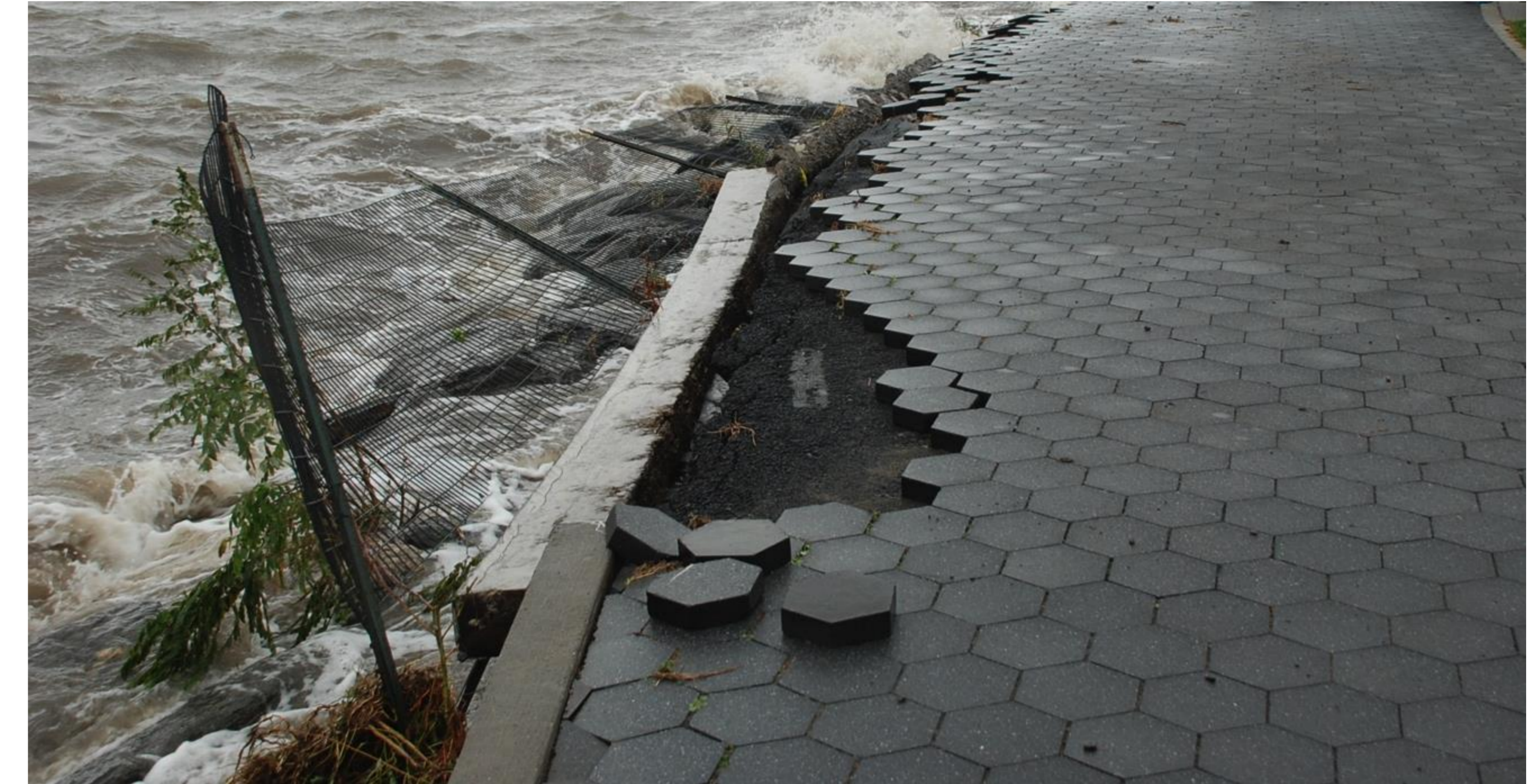
Eroded Shoreline (NYC Parks)
