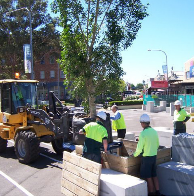
A one week installation period and a budget of AU$40,000 meant that innovation, collaboration and a lot of generosity needed to be shared to get the job done. Local government officers built new relationships and pride in their city.
