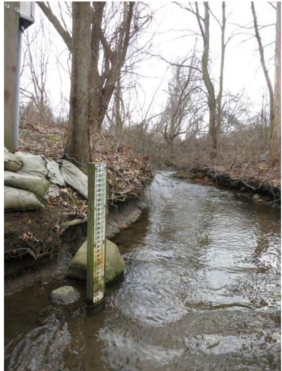
Alley creek - significant undercutting and invasive plants along the bank.
